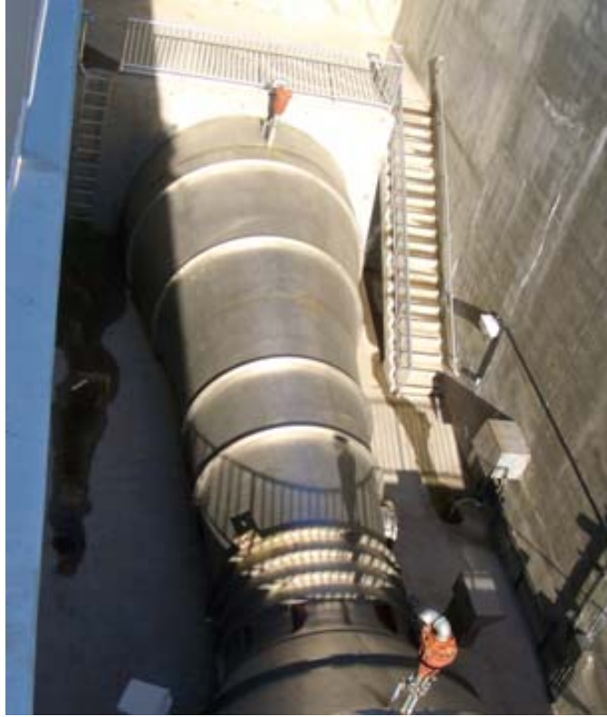
Figure 2: Venturi flow meter in a 15ft diameter water supply line near Lake Mead, Nevada.
