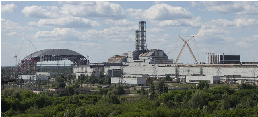
Figure 4: Cylindrical entombment structure (left) being prepared for installation over the damaged Chernobyl reactor (center). Photograph reproduced with the permission of the owner, Ingmar Runge.
